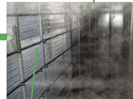
Project specific ecomist HVAC nozzle manifolds and glass fibre evaporation modules
